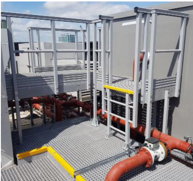
Ladders and Platforms
